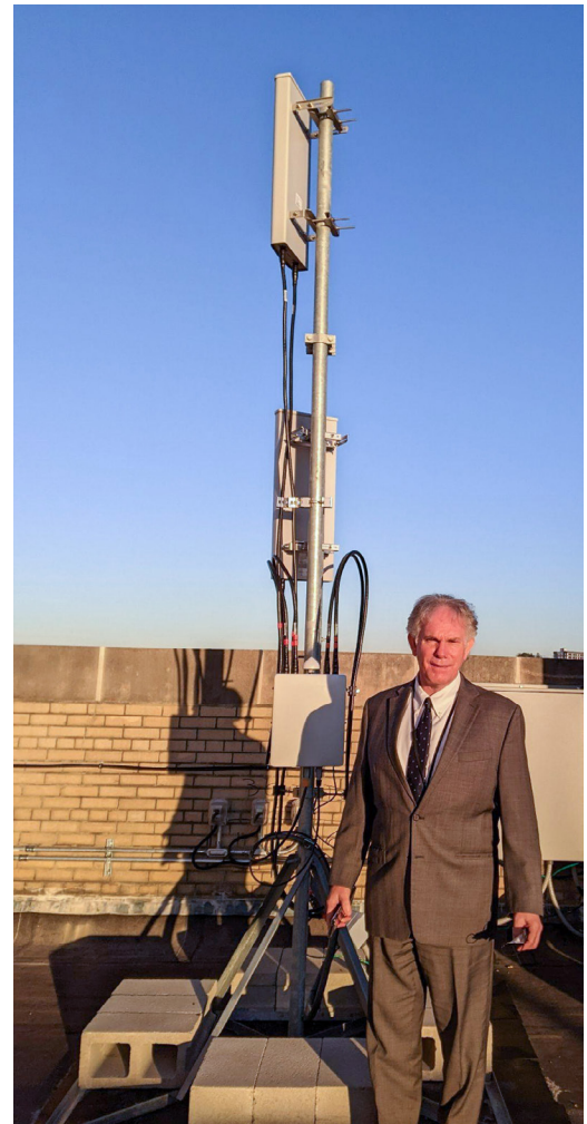
Pictured: Bob Cacace, CIO/COO, City of Yonkers, believes that the Infrastructure Investment and Jobs Act (IIJA) can help his city reach near 100% connectivity to all residents.
